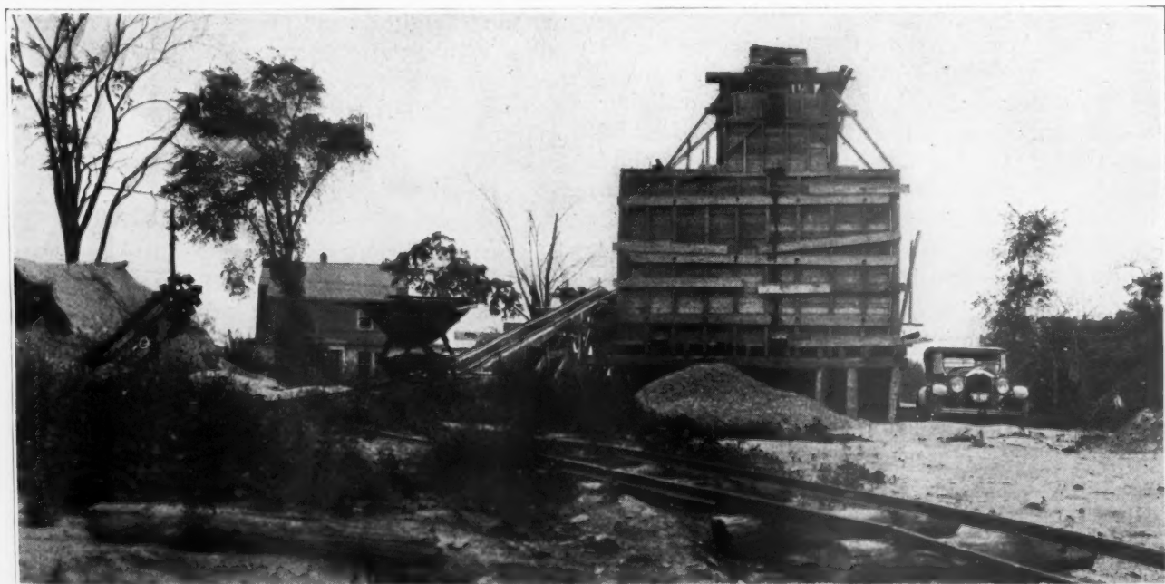
View of Incline to Crusher and Dump Car at Forgione and Romano.
